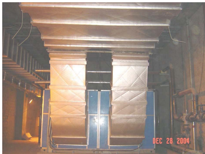
Platform Air Handling Unit
