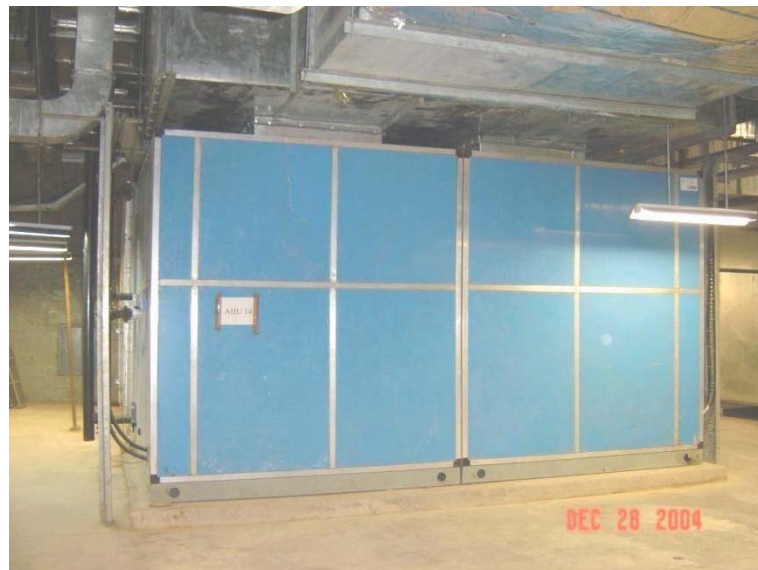
Concourse Air Handling Unit
